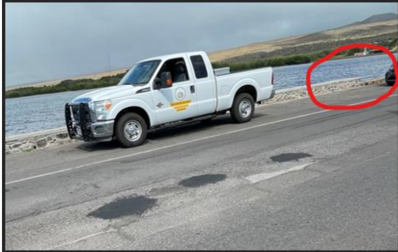
PHOTOGRAPH NO. 1: Junction of existing rock wall recently constructed and existing rock wall to be removed and reconstructed to match.
