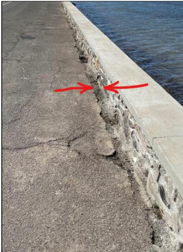
PHOTOGRAPH NO. 2: Existing asphalt pavement to be repaired along both existing and new rock wall.
